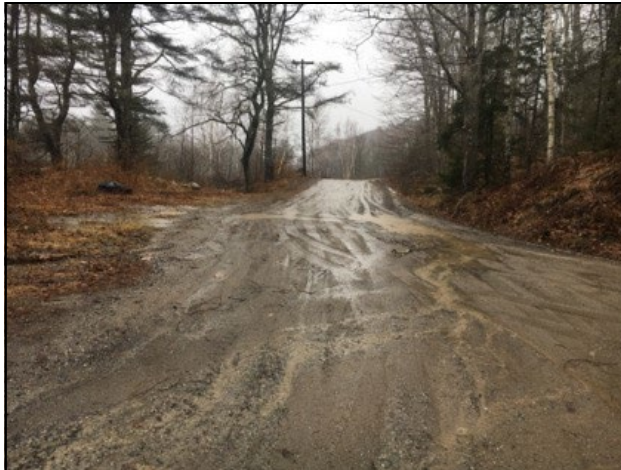
Gaecklin Road Before – The town road lacked stormwater BMPs causing severe erosion and polluted runoff.
