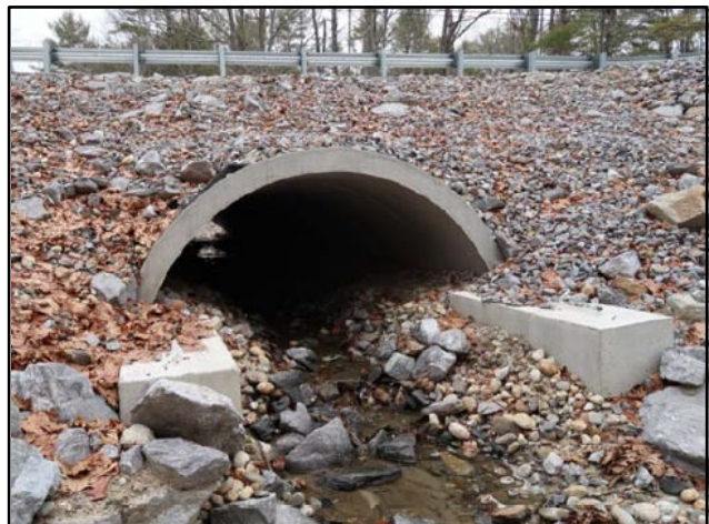
After – Downstream side of the crossing. More natural stream bottom under road, leading into created step-pools allowing for connectivity and for the energy to dissipate as it moves down the slope.
