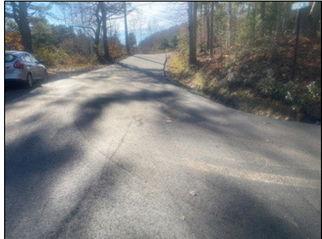
Gaecklin Road After – Various road BMPs were installed, which included paving, crowning, and ditching.
