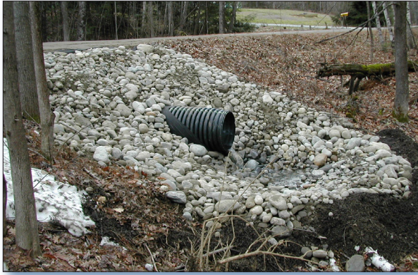
Figure 2. Adding BMPs reduced pollutant loading from gravel camp roads.
