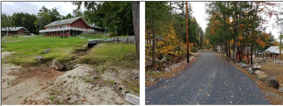
Pine Tree Camp before and after – Bluestone gravel was applied to 1,500 feet of chronically eroding road; 400 feet of ditch was stabilized; and two culverts were replaced and reset.
