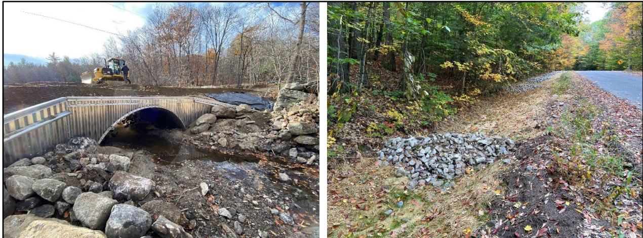
Sandy River Road – This steep road has had severe and chronic erosion problems for many years, and the crossing itself was undersized and collapsing. With funding from a State of Maine DEP Culvert Grant, Town of Chesterville and 319 grants, the site was able to finally be addressed with installation of numerous check dams, stabilized ditches, paved road surface, and a new aluminum, open-bottom arch culvert (22' span).
