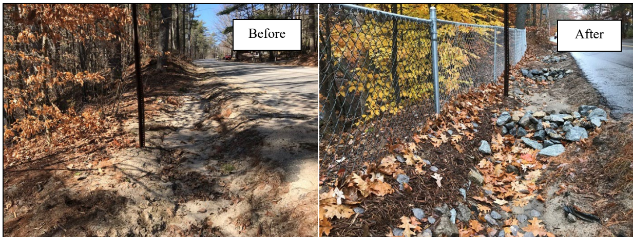
Pond Road – A steep, eroding path leading directly to the lake was blocked off with a fence and vegetated. An erosion control mulch berm was installed to direct stormwater from the road into an existing catch basin and check dams were added to the existing ditch.
