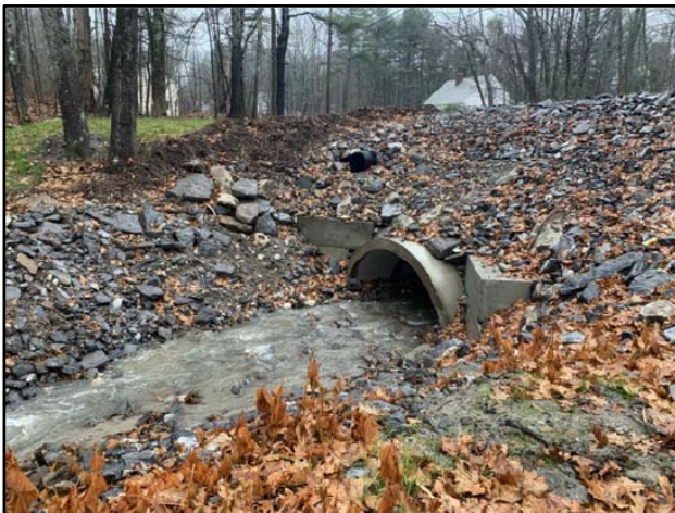
After – Upstream side of the crossing. Enlarged culvert removes constriction to the stream and allows channel to reform.
