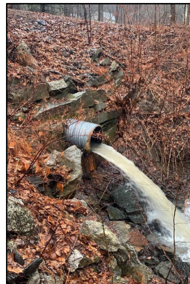
Before - The West St crossing. Stream was extremely constricted, disconnected and causing erosion downstream.
